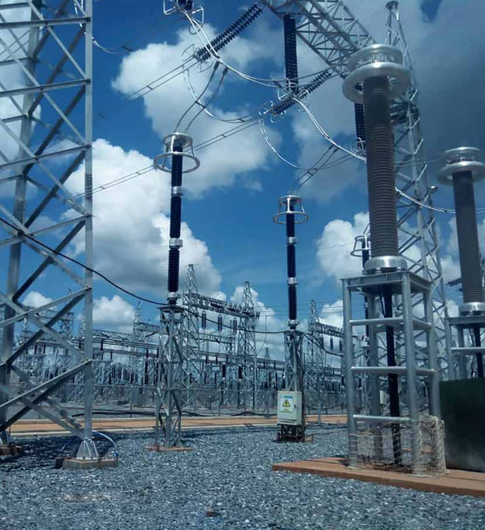
The 400kv Karuma Sub Station
